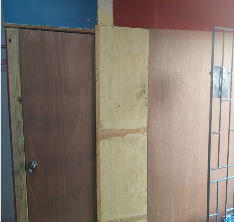
STORAGE AREA IN NEED OF PAINT
